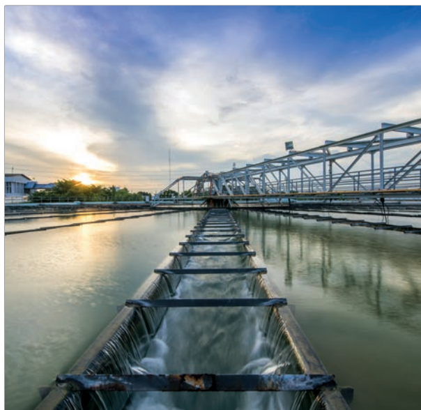
The Solid Contact Clarifier Tank type Sludge Recirculation process in Water Treatment plant
